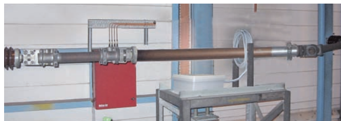
0.1% class Closed Loop F3 metering CT for DC valve hall
