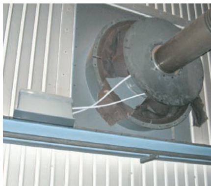
DC valve hall wall bushing
