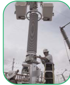
Bucket truck used to install 230 kV NXVCT system at Deer Valley Substation in Phoenix, Arizona.
