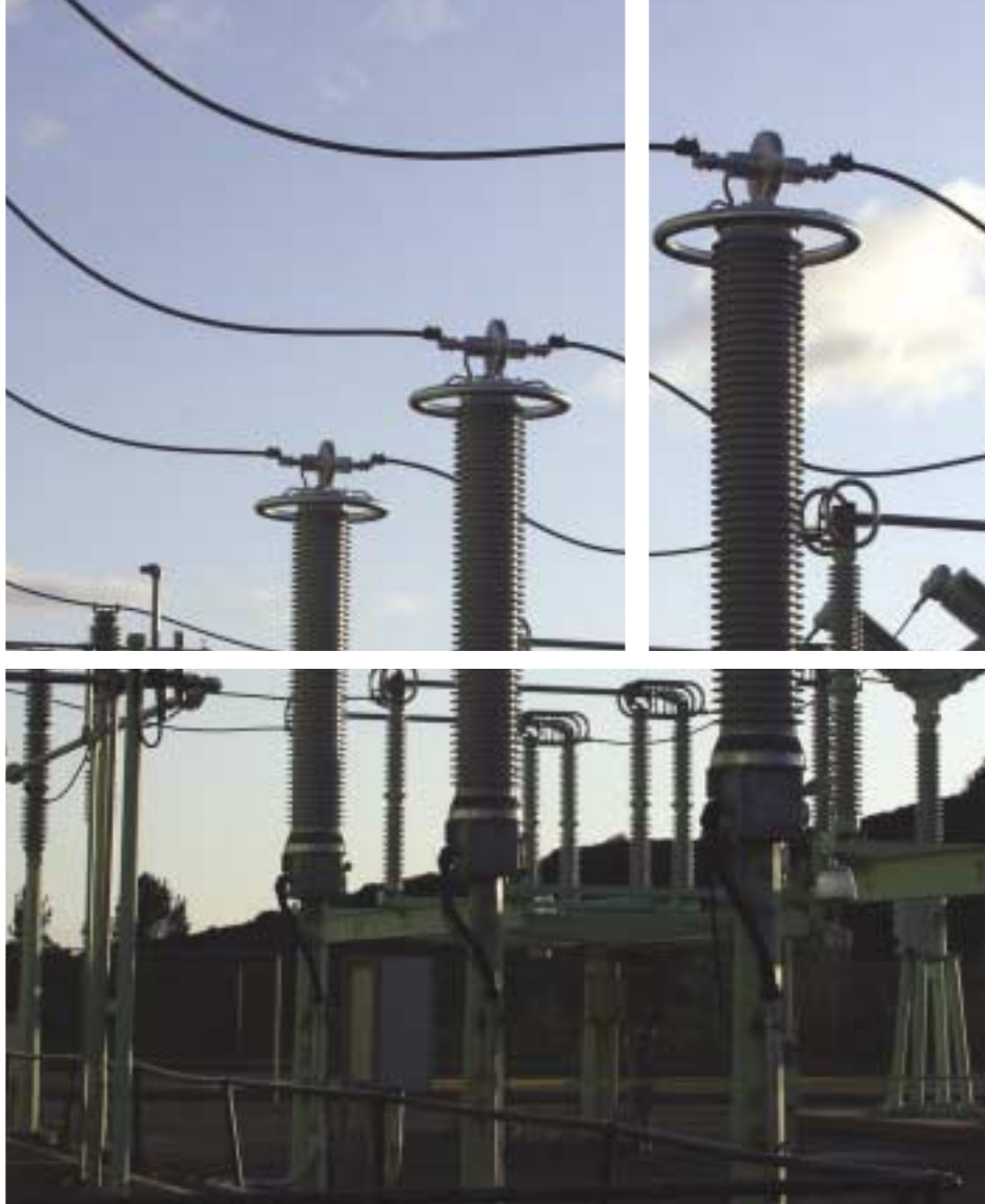
230 kV revenue metering system at Northern California Power Authority
